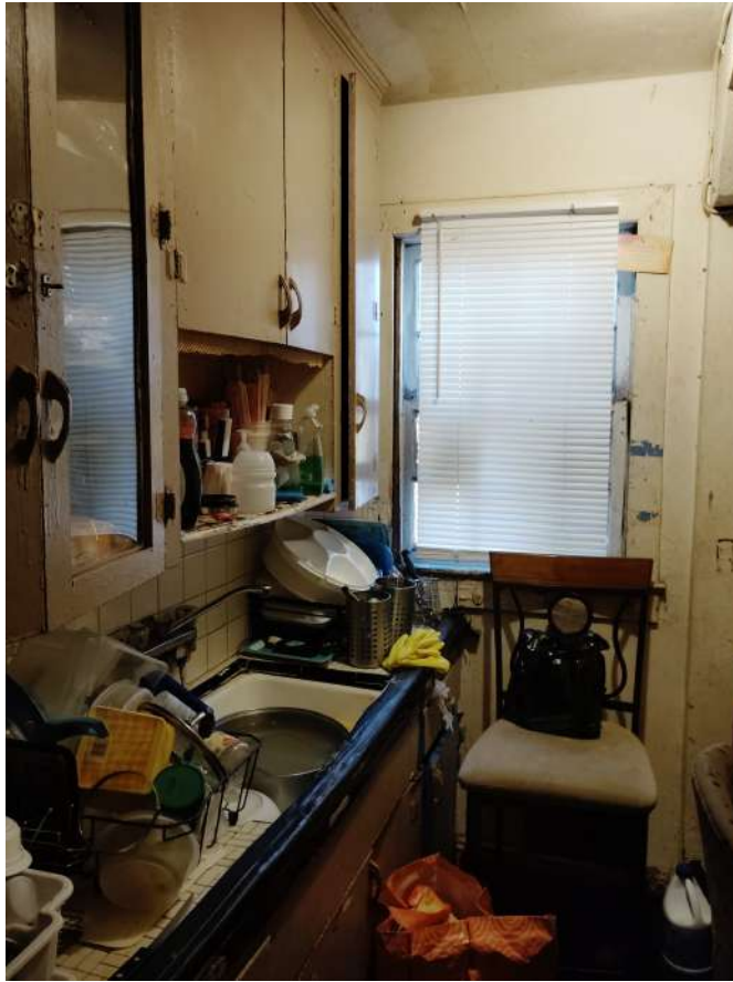
Photo: Kitchen: dated cabinets/finishes and signs of wear around sink/window
