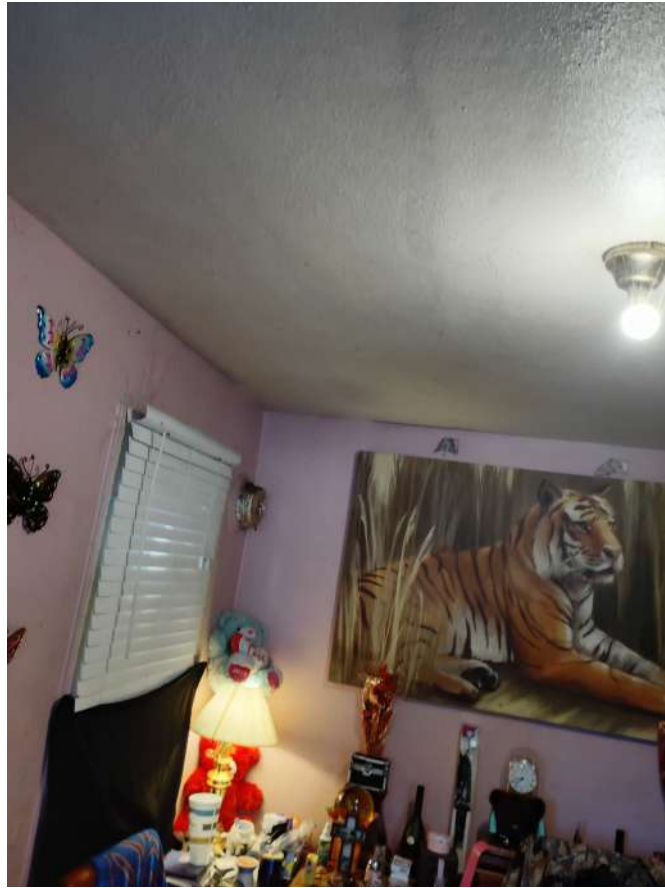
Photo: Interior ceiling: generalized discoloration; further moisture/mold screening recommended
