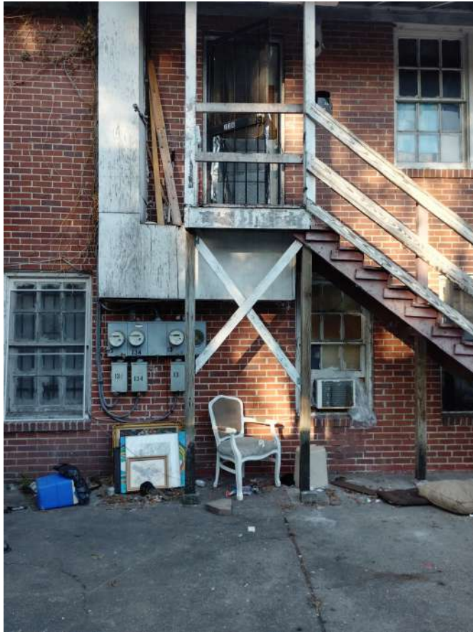
Photo: Meter bank and exterior framing: aged components, wood exposure
