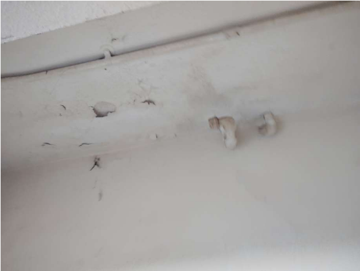
Photo: Interior ceiling: staining consistent with prior moisture intrusion
