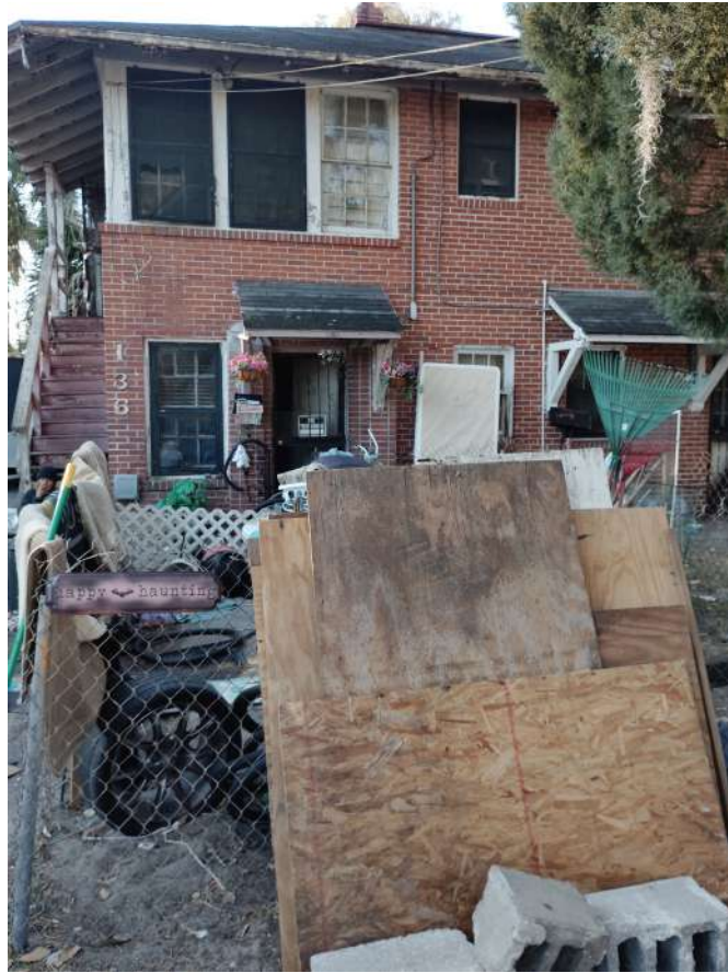
Photo: Front/side: site clutter, security concerns, aged windows/trim
