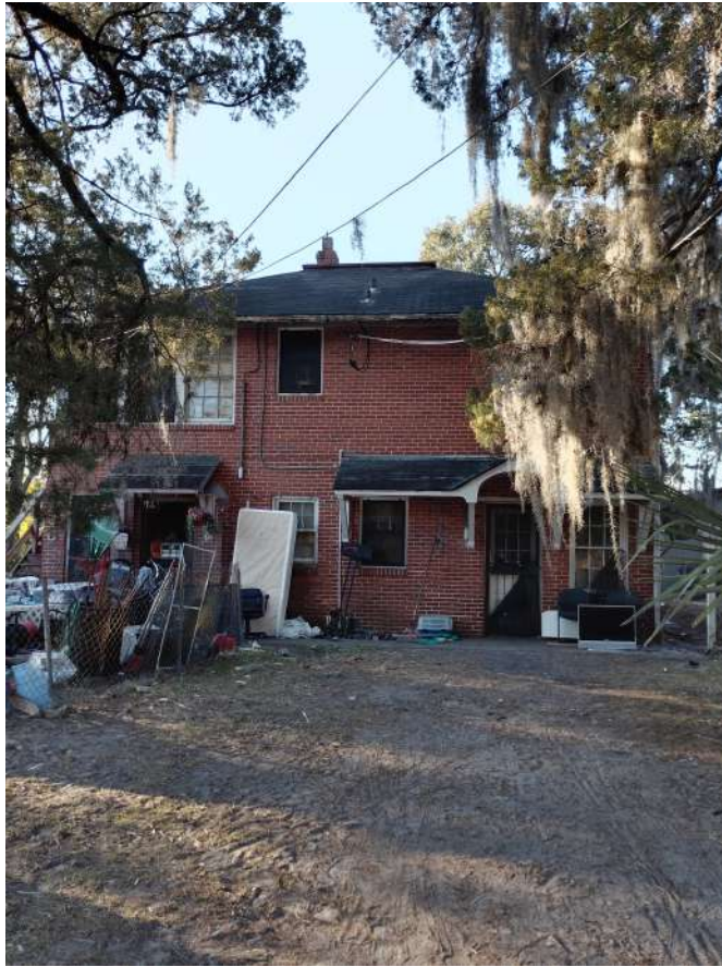
Photo: Front elevation: missing/broken upper windows and aged roof covering
