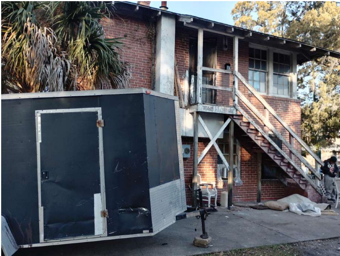
Photo: Rear/side elevation: exterior stair and balcony show deterioration
