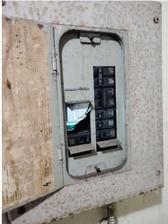
Photo: Electrical panel: corrosion and missing dead-front/cover plates observed
